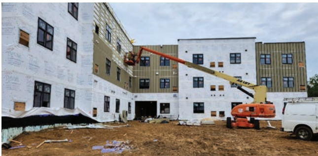
Workers used a crane to install siding on the main building in September 2022.
