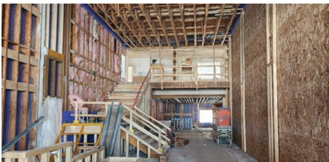
By year's end, the main building's two-story lobby was taking shape—a space that will welcome residents, visitors, volunteers, and staff to the campus community.
